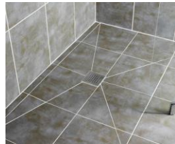
Shower Base Tiled Shower base
