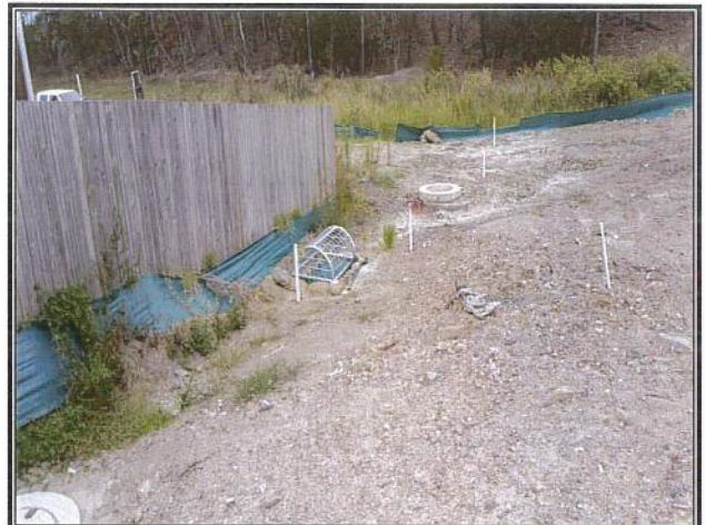
Sewer & stormwater on rear north side
